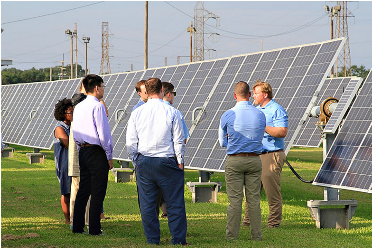
Master of Management in Energy students visit Entergy's New Orleans Solar Power Plant. (Photo courtesy Entergy Corp.)
